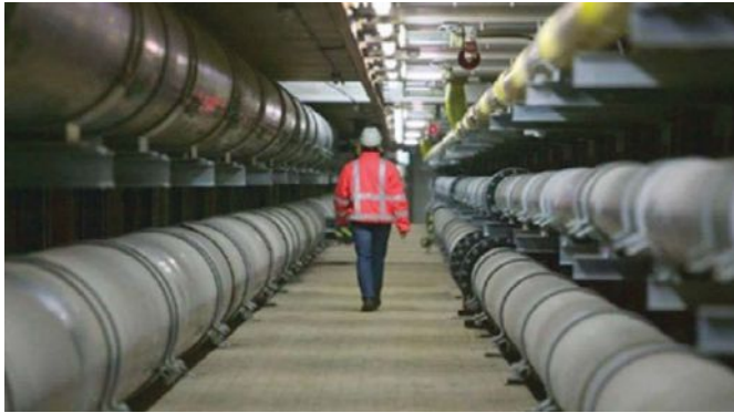
▲ Fig. 4 - Utilidor in Amsterdam carries multiple utility lines SOURCE: Courtesy H. Admiraal.
