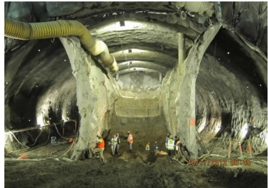
Figure 1 - Multiple drifts and ground freezing allowed successful SEM construction of Northern Blvd Crossing in New York
