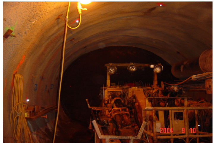
Figure 2. NATM tunneling at west utility building tunnel and installation of initial tunnel support.
