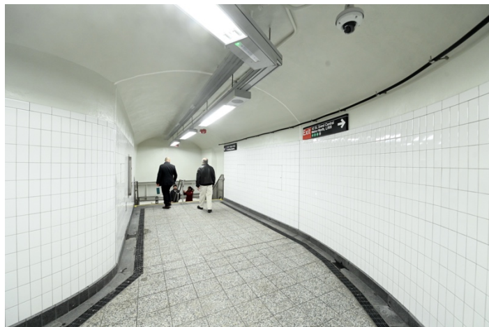
Figure 2. Completed new passageway connecting from the wall of the existing walkway going towards the Flushing Line at the platform level (Image Courtesy MTA).
