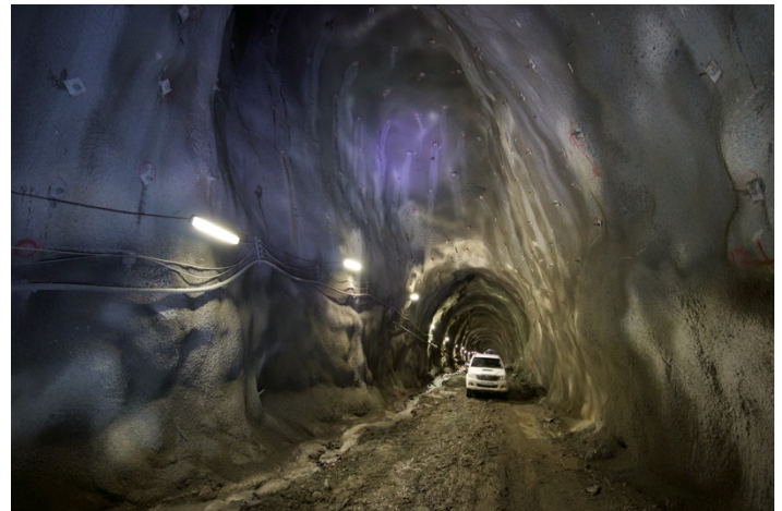
Figure 2. Repaired section of major rock fall.
