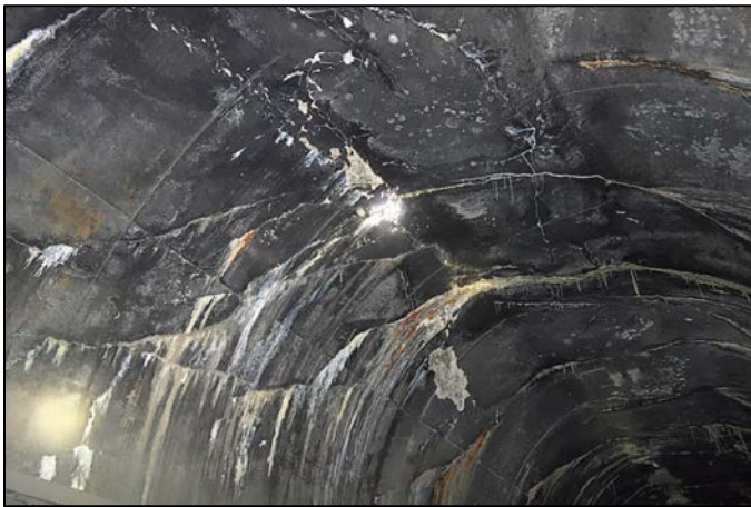
Figure 3. Typical damages in the tunnel's back.
