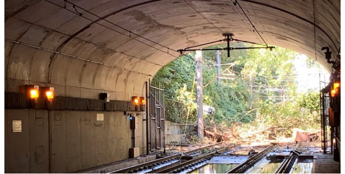
Figure 1. View of track from within the Weehawken Tunnel after debris flow at the West Portal.
