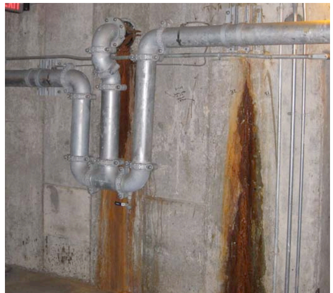
Figure 2: Tunnel leakage in construction joints
